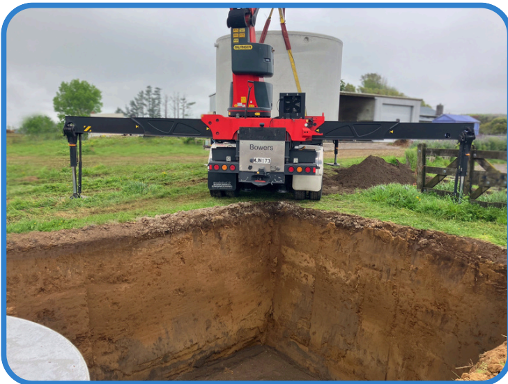
Example of the correct truck position for unloading into the prepared site.
