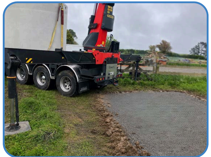
Example of the correct truck position for unloading onto the prepared site.
