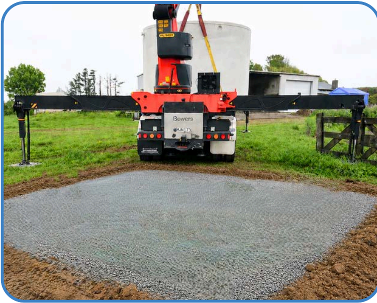
Example of the correct truck position for unloading onto the prepared site.
