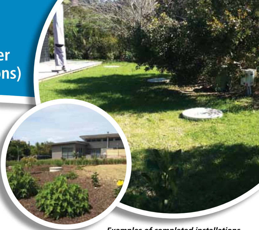
Examples of completed installations
